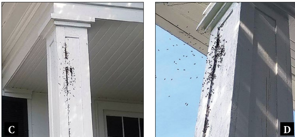
Figure 5. Here are several established honey bee colonies in cavities of a single house. A. Older homes tend to have more access ports for bees because of natural decay and settling of wooden structures that allows cracks and crevices to form. B. Staining of the wood identifies the entrance bees used to get behind the siding of the house to their colony in the hollow wall behind the façade. C and D. A colony of bees used this entrance to the tall, hollow columns of the porch. (Photos by J. W. Harris)
